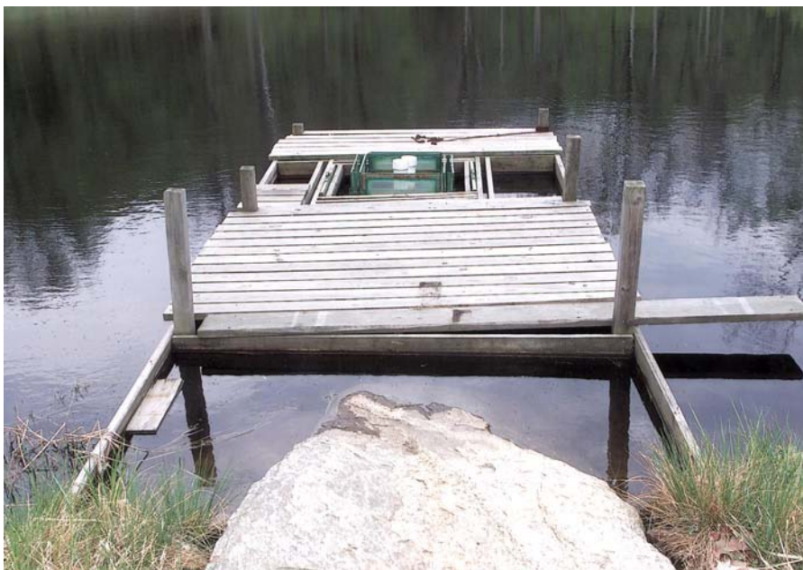
The intake pipe is secured to the bottom half of a new septic tank hidden beneath the dock.
