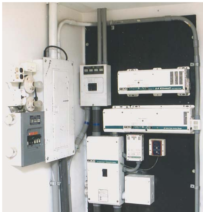
In the power room, hydro and solar power converge. When the batteries are full, excess hydro or solar electricity is used to heat domestic water.
