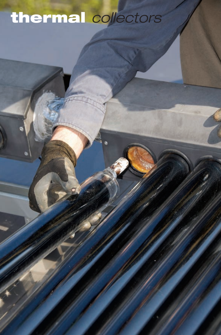
Individual evacuated tubes connect into a manifold.
