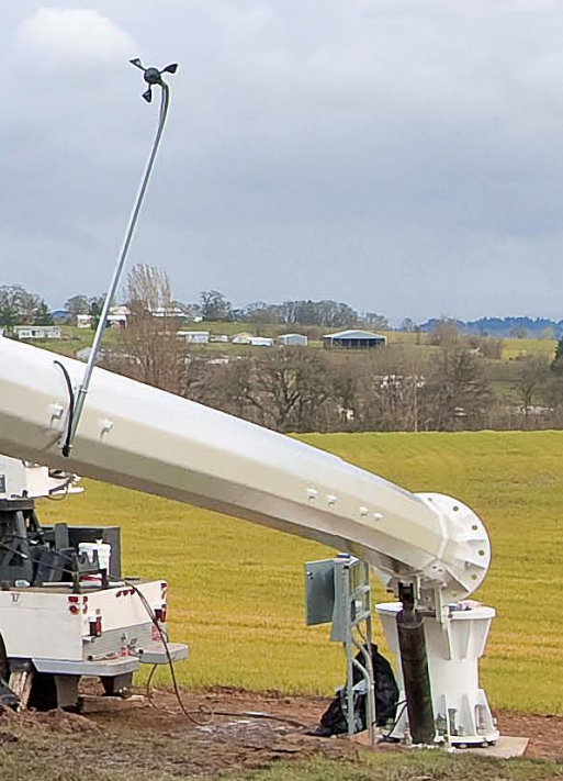
Tilt-up towers require a large, open site to raise and lower the tower, but guyed towers can be sited on cluttered sites and even between buildings.
